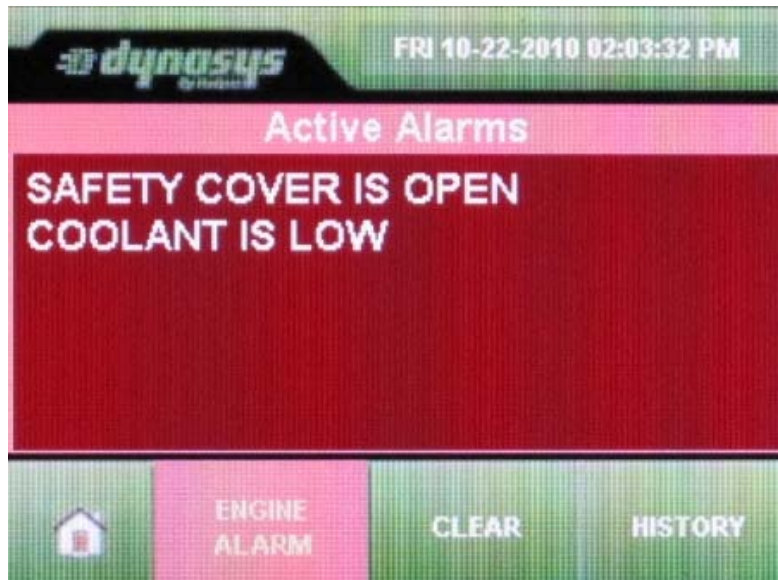
Figure 7 Active Alarms Screen
